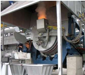
\ FARD rotary furnace
